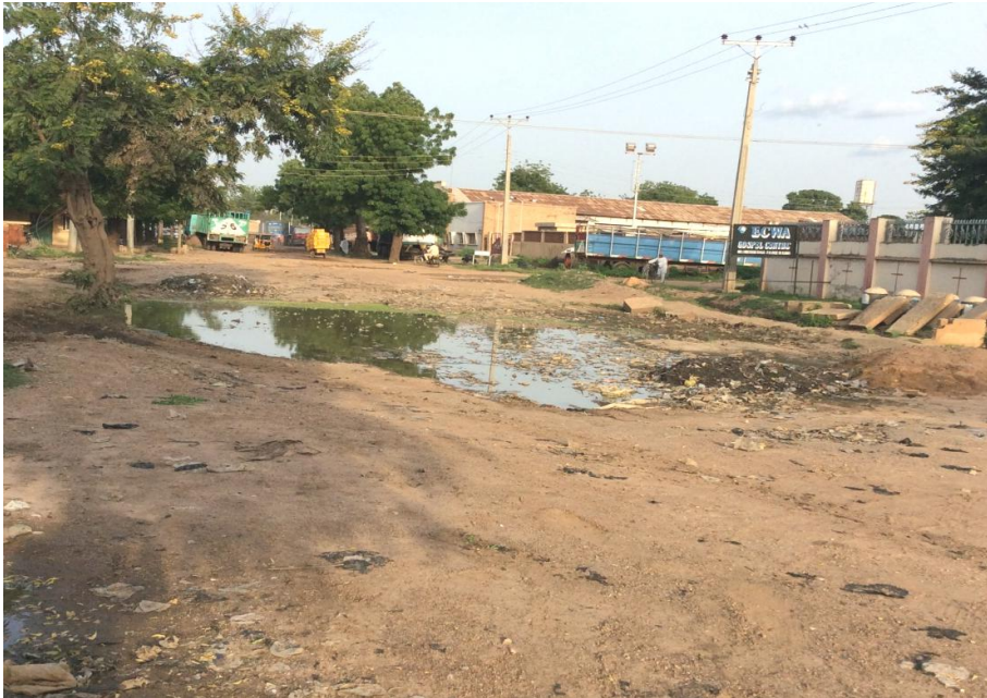
Plate 2b: Failed road in Bompai Industrial Estate, Kano (Aug. 25, 2017)
