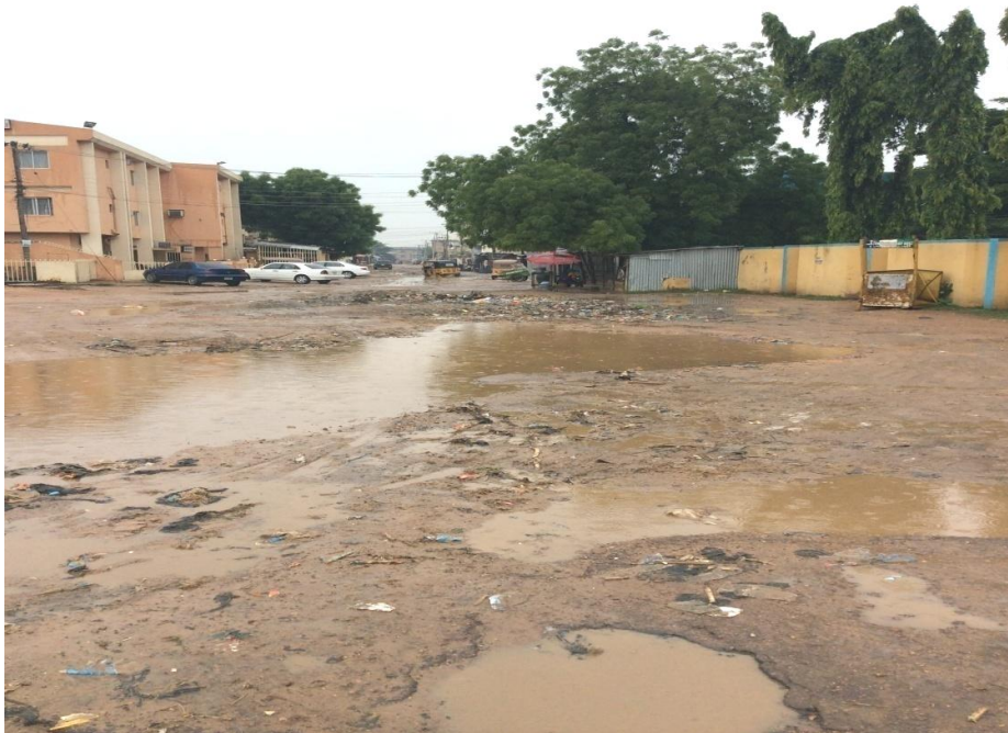
Plate 2a: Failed road in a well planned Nomansland residential area in Kano (Aug 30, 2017)
